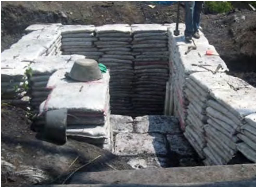
Construction of the trap using sandbags which if not lined with CC, would eventually degrade due to water erosion and UV degradation
