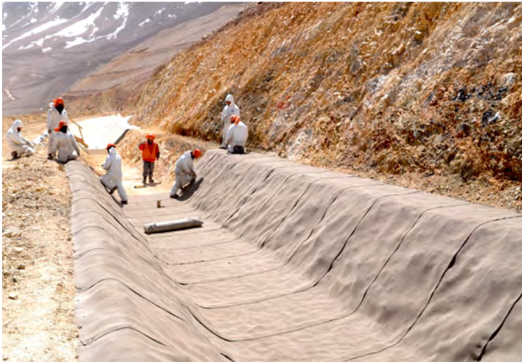
CC pegged to head of ditch edges and buried in anchor trench
