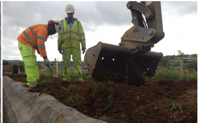
The edges of the CC were anchor trenched and backfilled after hydration.
