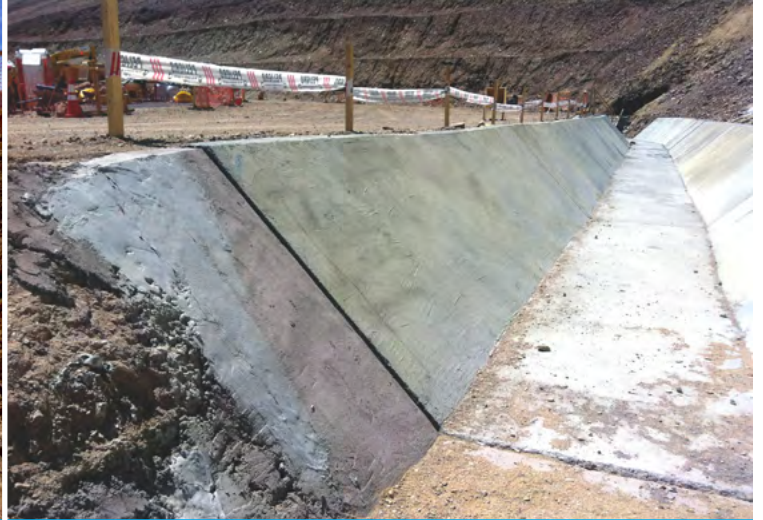
Parts of the ditch had been lined using poured concrete in the past
