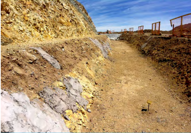
The ditch was graded and cleared of rocks and debris prior to installation
