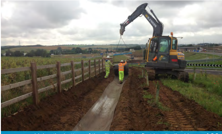
Lining the bottom of the ditch with the first longitudinal layer of CC
